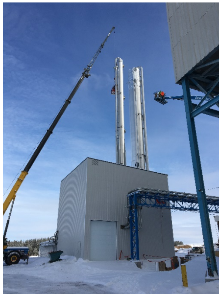
CO 2 Solutions 30 tonne-CO 2 per day carbon capture unit under construction in Saint-Félicien, Québec.
